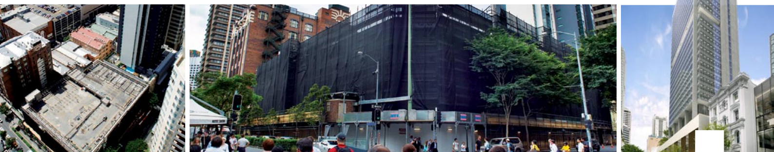
Above: Construction is underway at 123 Albert Street, Brisbane QLD (left and centre) and an artist's impression of the completed office tower (right)
